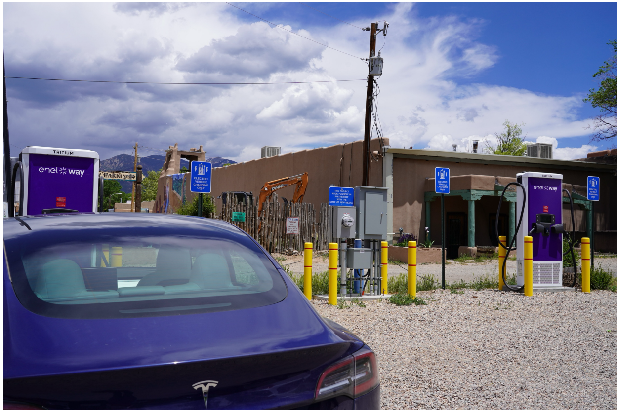
Pictured: KCEC DC level 3 EV fast chargers are adjacent to the Taos Plaza in Taos, NM. KCEC has 36 EV chargers with 58 charging points in its service territory.
